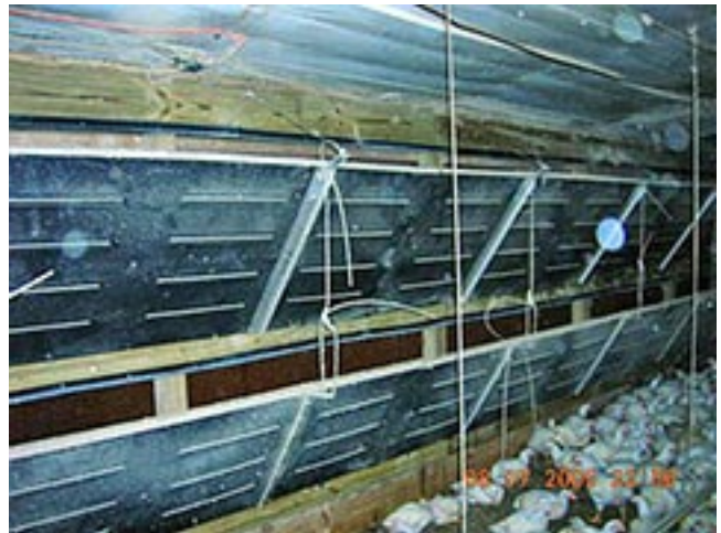
This photo of a tunnel inlet door system in open position shows how the doors direct airflow upward as it enters the house, which helps eliminate dead air spots commonly seen with tunnel inlet curtain systems. A possibly serious drawback with this system is that it does not allow knee braces, which may be needed to protect the structural integrity of the house.
